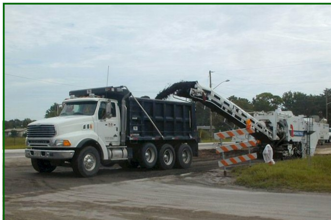
Milling Asphalt Pavement for Recycling (from Reynolds, Smith, and Hill CS, Inc.)
