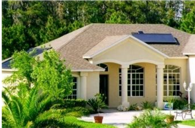
Figure 7.1 Active Residential Solar Thermal Collector (FlaSEIA, nd)
