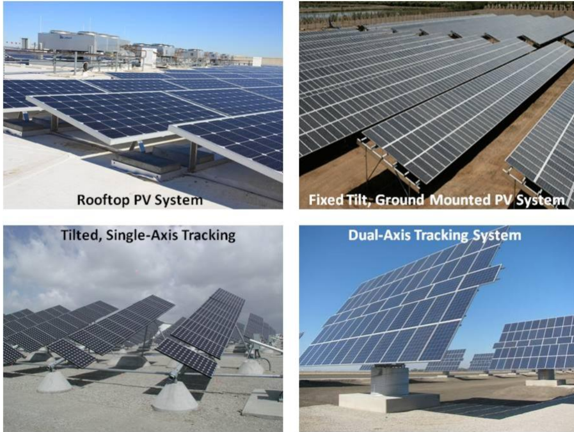
Figure 4-1 Example Solar PV Installations
