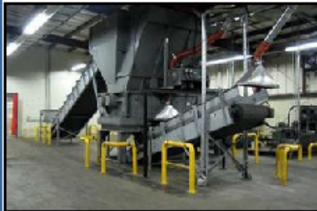
SRS Shredder in Salley, SC
