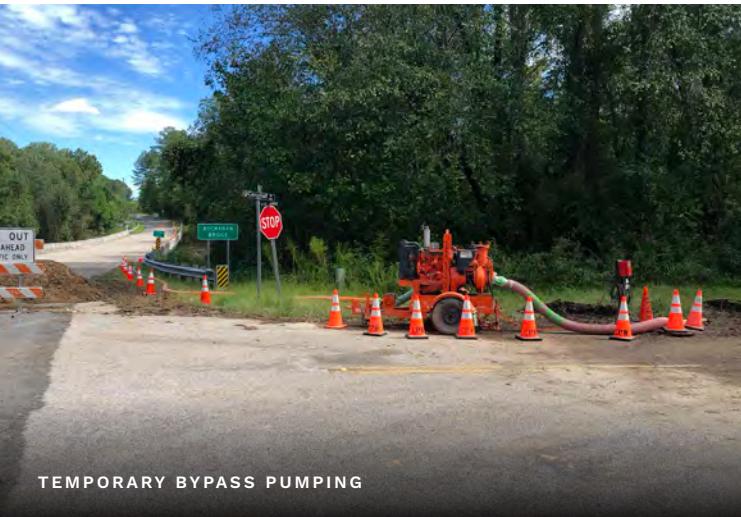
COLLAPSED SEWER LINE
